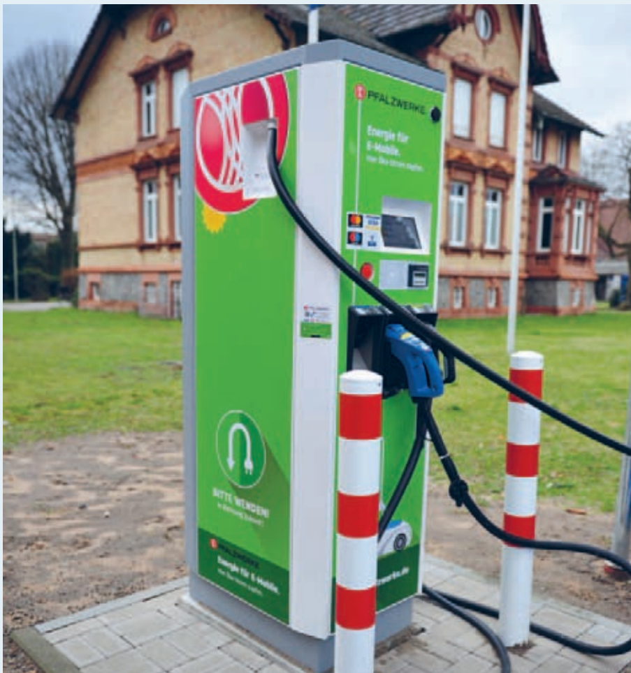
Supported charging station with protective posts
