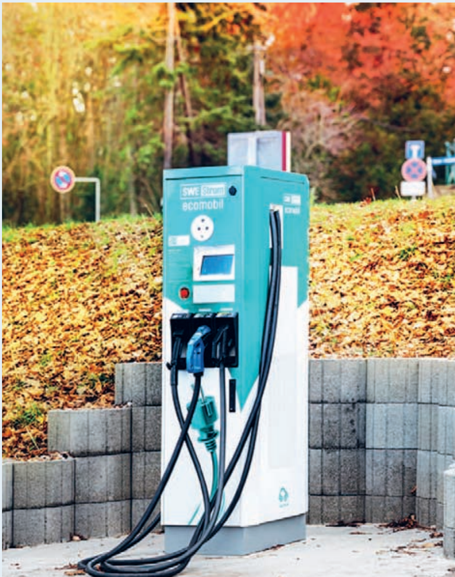
The Thüringenhalle charging station
