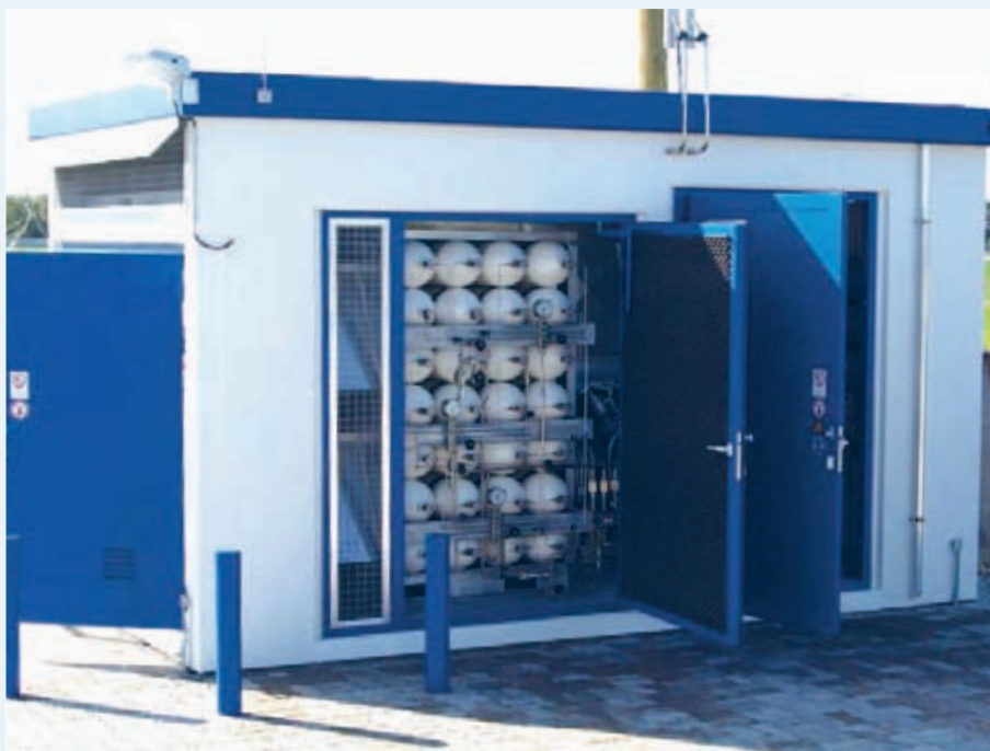
Building at an H 2 filling station with high pressure storage and compressors
